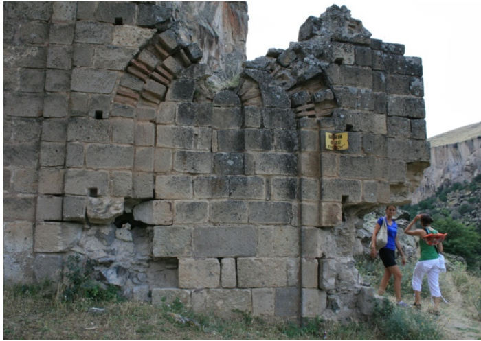
Fig. 34: St. George church (Karagedik Kilise), Peristremma (Belisırma), Cappadocia, continuous wooden reinforcement below the window sills (July 2009)
