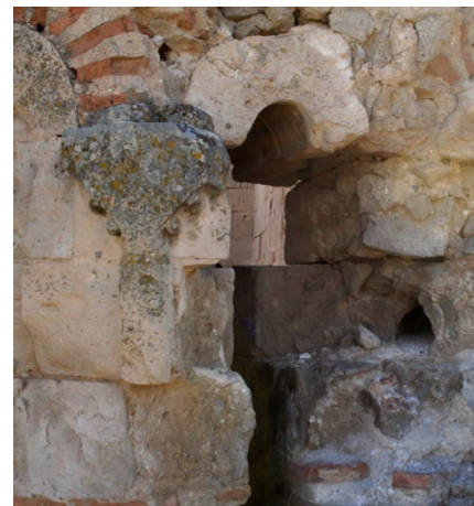
Fig. 41: Çanlı Kilise, Aksaray, Cappadocia, continuous wooden reinforcement at the springing of the main window arches, east façade (July 2009)
