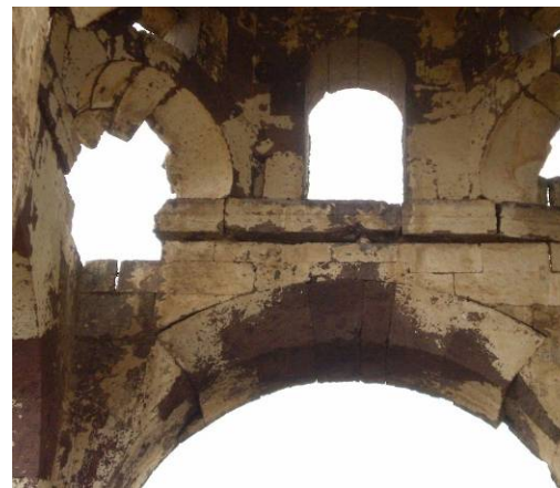
Fig. 28: Kizil Kilise, Cappadocia, interior view showing traces of the wooden reinforcements at the base of the dome drum and squinches (July 2009)
