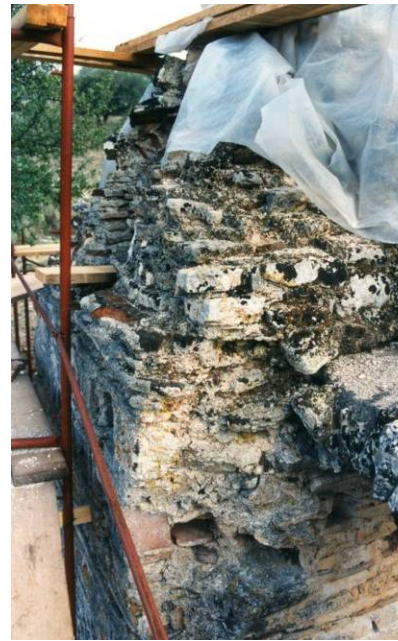
Fig. 13: Hagios Stephanos, Rivio, , traces of wooden reinforcements at the springing of cross-arm barrel vaults (Mamaloukos and Kamboli 1995)
