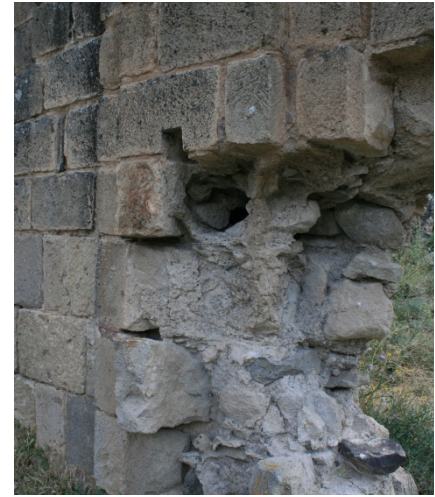
Fig. 35: St. George church (Karagedik Kilise), Peristremma (Belisırma), Cappadocia, closeup of wooden reinforcement and putlog hole below the window sills (July 2009)
