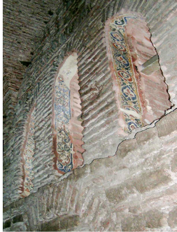
Fig. 38: Zeyrek Camii, exonarthex, windows in north wall with surviving wooden beams at mid height (Ousterhout et al 2010, Fig. 18)
