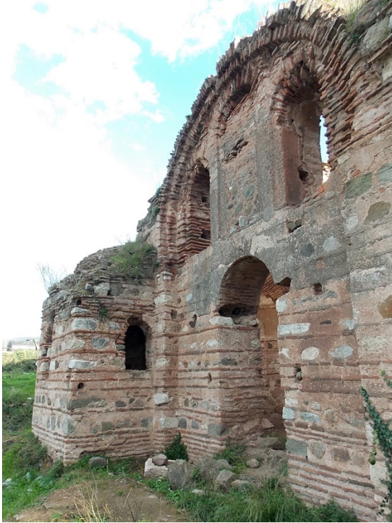
Fig. 37: St. Abercius church, Kurşunlu (Elegmi), Bithynia, staggered connection between exposed beam and built-in wooden reinforcements (three more wooden reinforcement systems, one below and two above, are also discernible) (March 2013)
