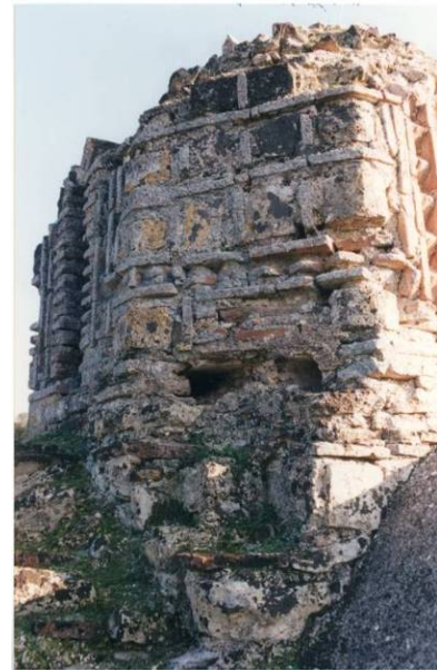
Fig. 24: Hagios Stephanos, Rivio, , traces of wooden reinforcements at the base of the dome drum (Mamaloukos - Kamboli 1995)
