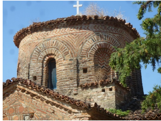
Fig. 26: Mary, Kosinë, Albania, view of wooden reinforcements at the base of the drum on the exterior (September 2014)
